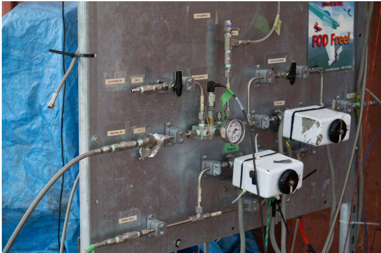
Figure 135: Assembled Nitrous Oxide Panel
